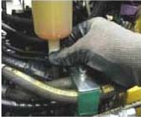
Water Drain Valve
